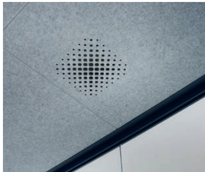
Fresh air is drawn into the room via an invisible sound absorber integrated in the acoustic ceiling
